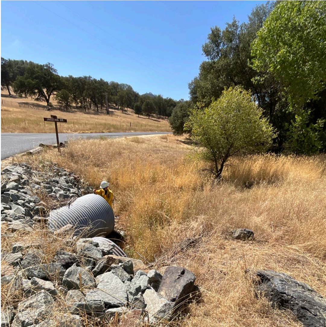
Figure 9. Photographs of VAR #4 showing inlets of two 60" culverts. There was evidence that flooding had previously occurred at this location.
