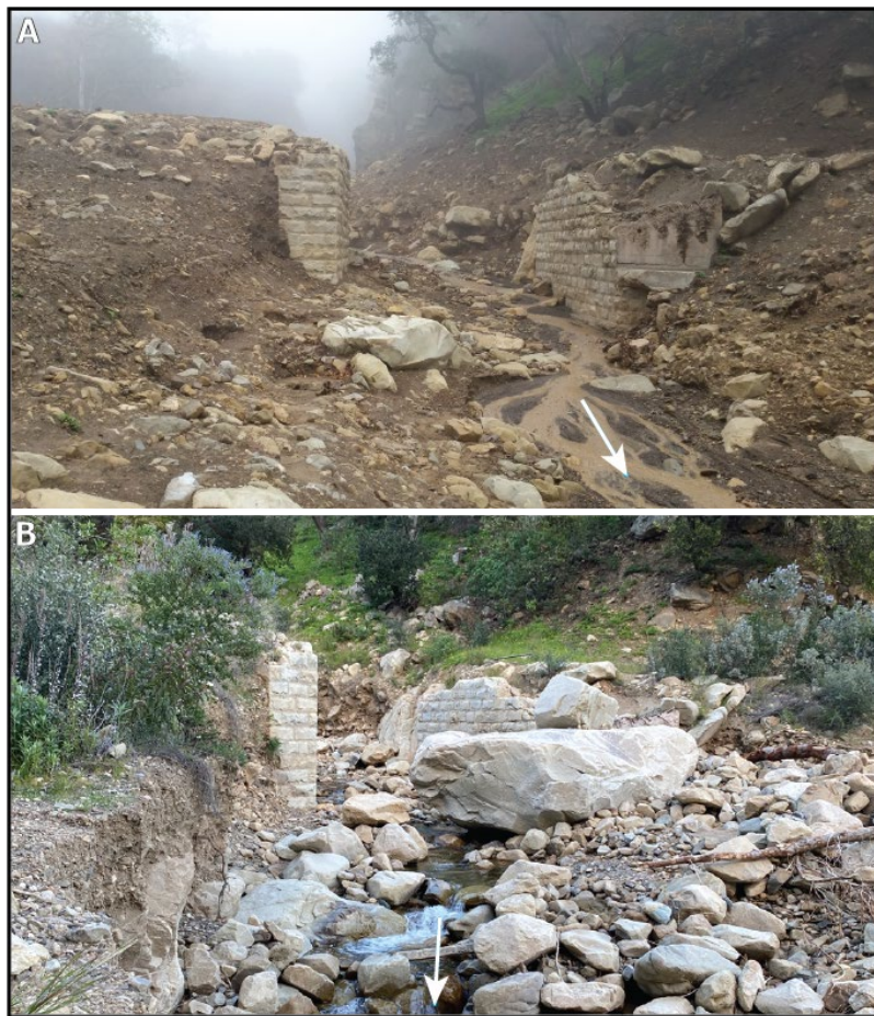
Figure 10. A. Before photo of bridge abutments in Romero Creek shortly after 1-9-2018 debris flow event. B. After photo following 1-9-2023 flood of bridge abutment showing aggregated alluvium downstream. For scale, the large boulder in (B) is approximately 15 feet wide. Arrows in the photos indicate flow direction.
