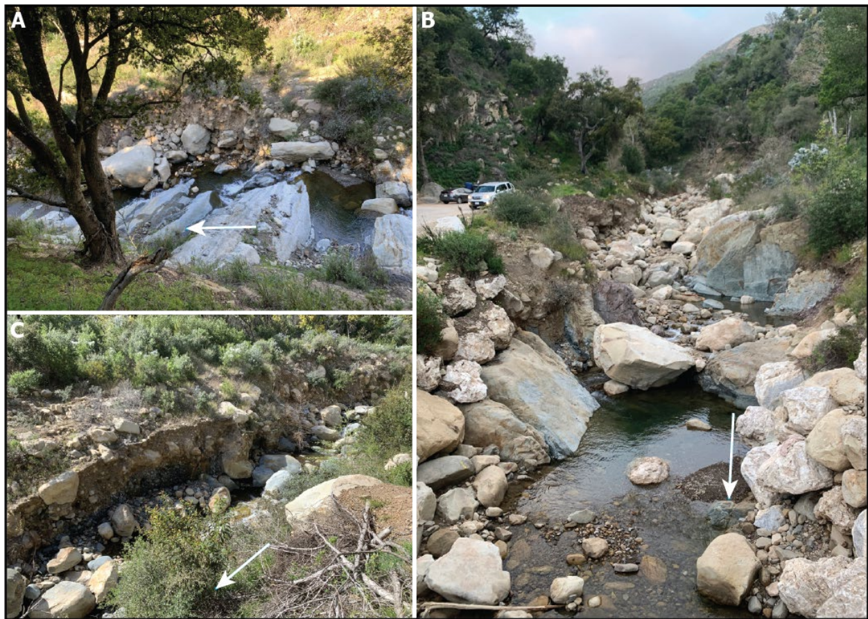
Figure 9. Amount and distribution of available sediment throughout the mainstem channels. A. More evidence of scour within mainstem channels than deposition in San Ysidro and (B) Cold Spring Creeks. C. Easily erodible sediment currently located in mainstem channels is available to transport in San Ysidro Creek. Channel widths are approximately 50 ft (A and B), and 30 ft (C).
