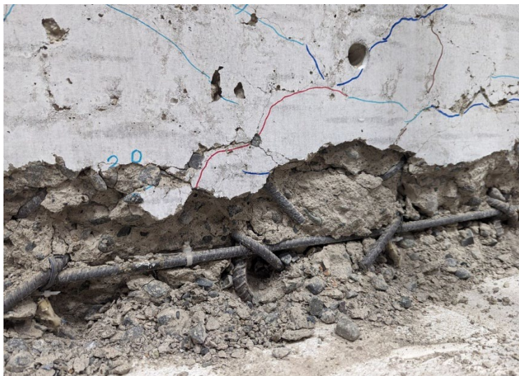
Figure 8. Sliding interface of Wall 3 after the test. The vertical bars are kinked.
