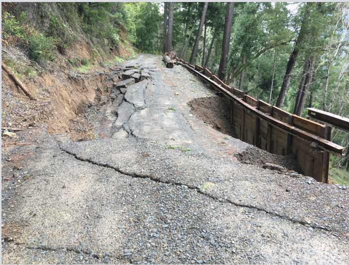
Roadway affected by a landslide that can be repaired, though it may require a long closure and additional engineering work.
