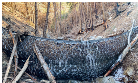
Debris nets stop rock and debris.
