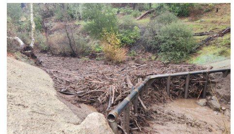
Debris racks stop rock and debris. Photo: Matt Griffin.
