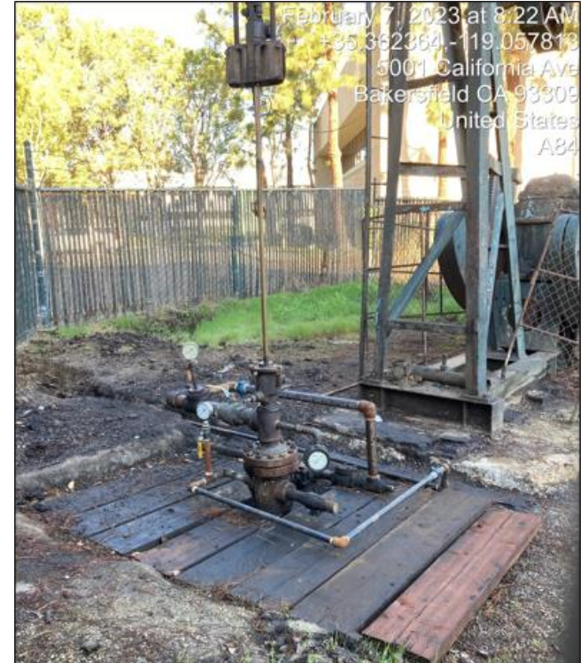
Well that leaked gas in Bakersfield (Summer 2022)/ Pozo con fuga de gas en Bakersfield (verano de 2022)
